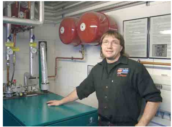
Stefan Bleyer uses an eco-friendly block unit heating power plant for heating.
